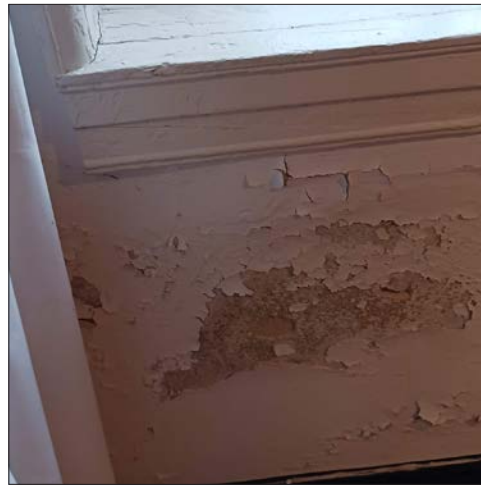
78-1: Peeling of plaster and paint below window.
