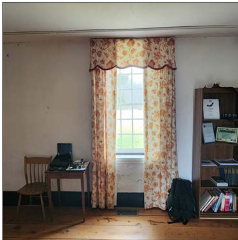
78-3: Significant damage to plaster under windows
