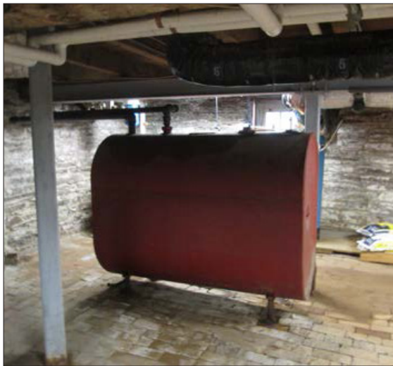
108-2: Fuel oil storage system
