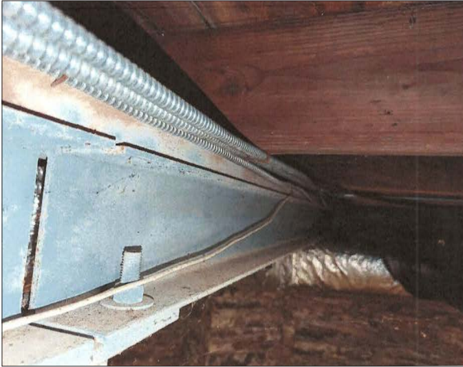
104-1: Rows of steel beams have been added at midspan of the first floor joists.
