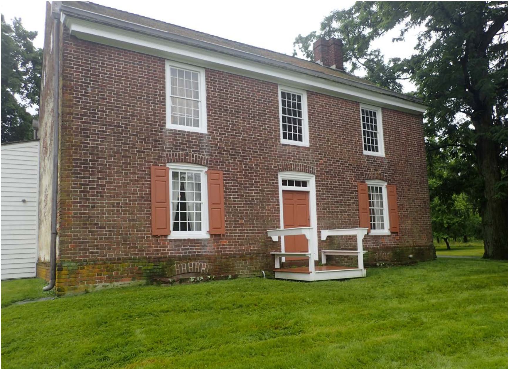
153-1: Immediate recommendations include cleaning of mortar and bricks, repointing mortar, and patching masonry.
