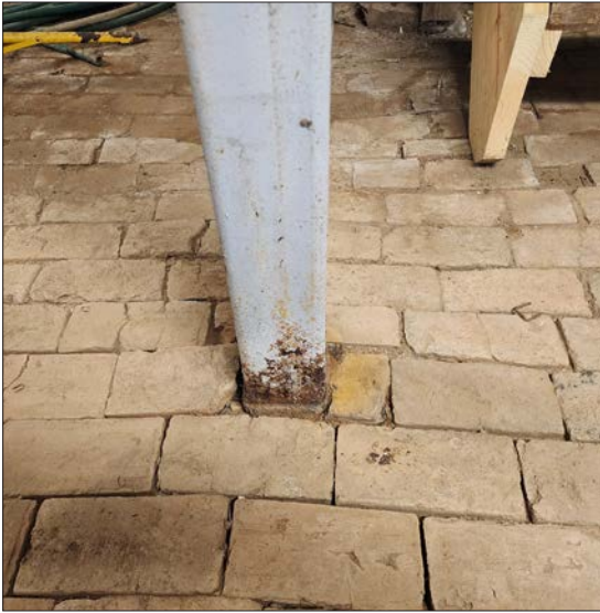
152-1: Corroded steel columns
