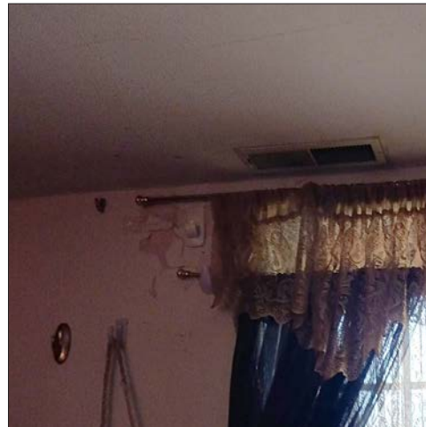
91-5: Failing plaster around window indicates possible water infiltration.
