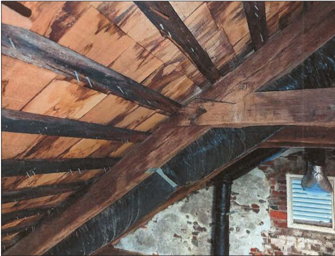
104-3: The roof framing is in good condition and is adequately supporting anticipated gravity and lateral loading conditions.
