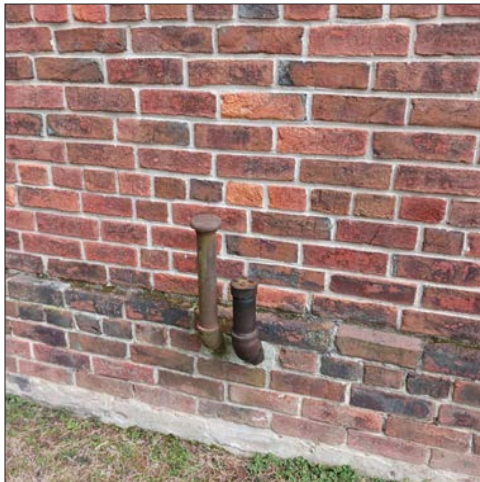
54-3: Pipes protruding from wall. Bricks in wall are spalling and cracked.
