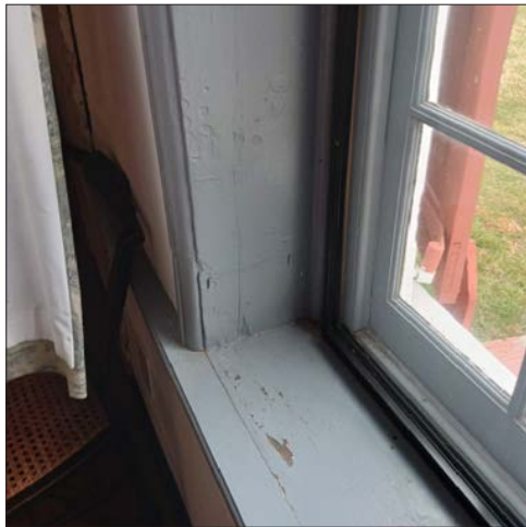
73-3: Paint at windowsill and jamb is peeling.
