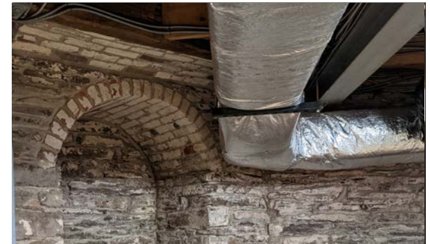
109-1: First floor fan coil and distribution ducts
