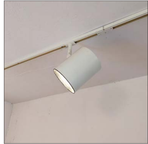
98-3: Track lighting dates to 1999.
