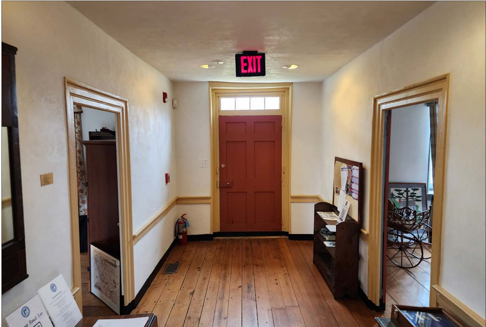
69-1: First floor corridor has exit signage, thermostat, lighting, and required fire alarm pull.
