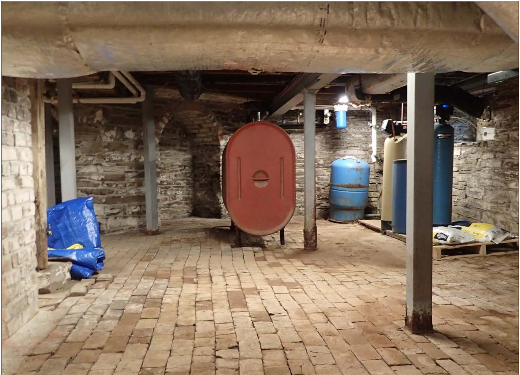
60-1: Building systems equipment, including oil heating and well water systems.
