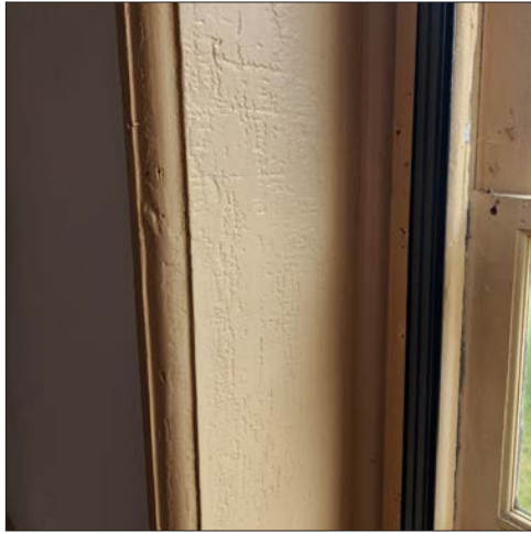
98-1: Scratches and damage to window frame
