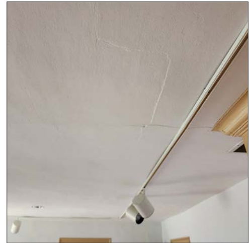
98-5: Cracks in ceiling plaster.
