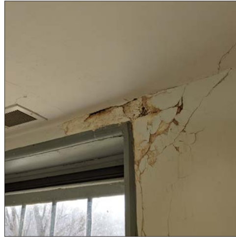
94-2: Cracked and peeling plaster around window head and ceiling.
