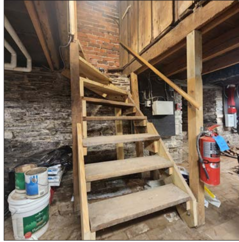
59-5: Steps from basement to first floor. Treads and stringers appear to be recently replaced.
