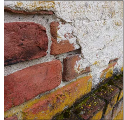
50-2: Spalling and damaged bricks, coating should be cleaned and examined further.
