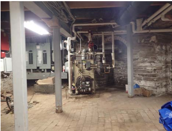
148-2: Address columns at basement level to prevent further corrosion
