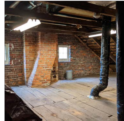
101-5: View of gable end and chimney showing spalling of bricks.
