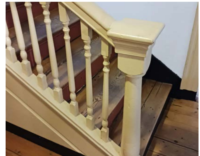
143-2: Existing historic handrails may remain even when they do not meet code requirements for new construction.
