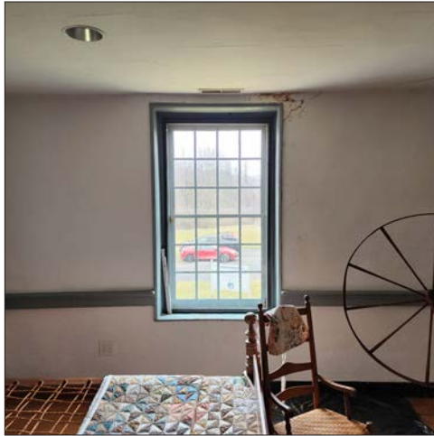
94-1: Cracked plaster ceiling and walls.
