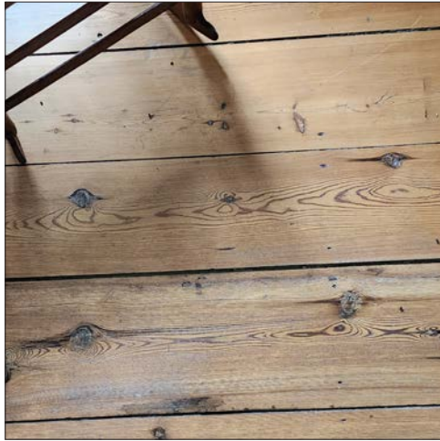
64-1: Original wood flooring exists throughout the house and should continue to be maintained.
