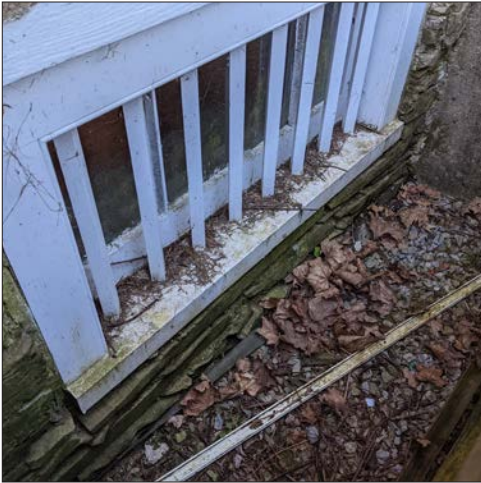
39-1: The window wells are clear of vegetation, and should continue to regularly be cleared of leaves and debris. Moss is growing on various surfaces.
