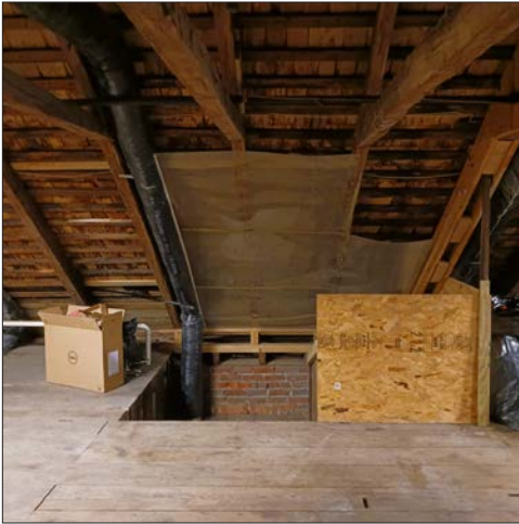
101-1: Stairway to second floor. Plastic sheeting has been installed to the roof joists.
