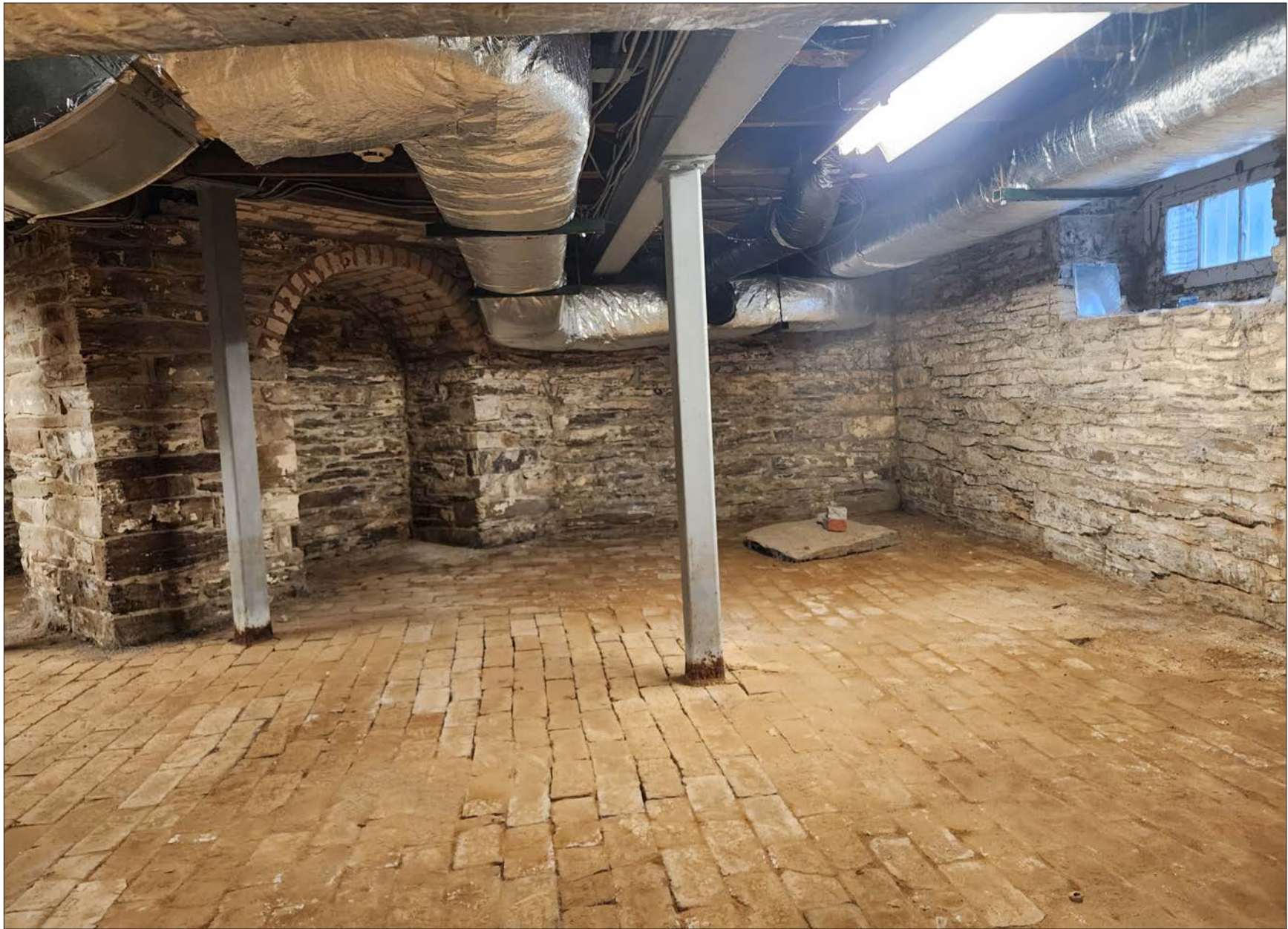
61-1: Existing view of rubble masonry walls and contemporary interventions including steel supports and mechanical ductwork. Flooring is generally dry with sporadic locations and periods of water infiltration.
