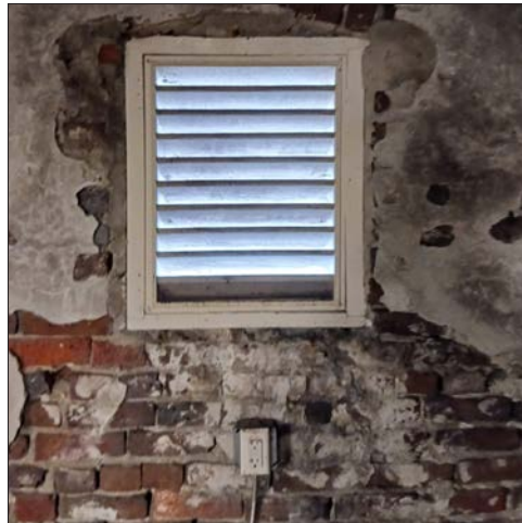
101-4: Louvered opening and electrical outlet.
