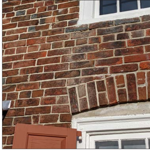
46-5: Mortar and brick condition at South elevation.
