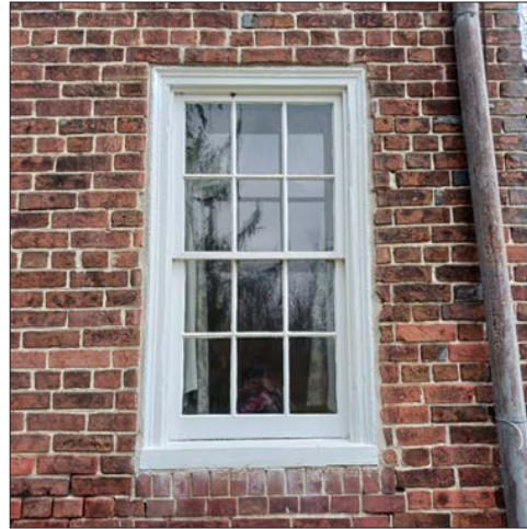
54-2: Efflorescence at window and some spalling bricks around window. Note areas of mortar loss at lower left of image.
