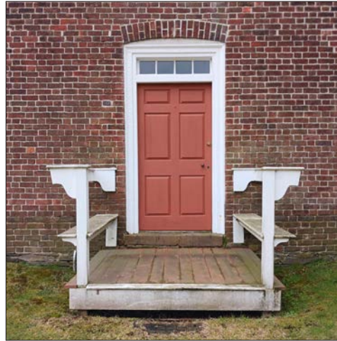
39-2: Porch has become dirty over time, porch and benches are in stable condition.
