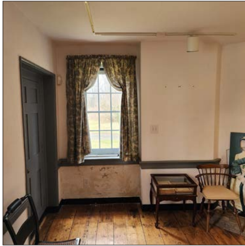
73-1: Significant damage to plaster below windows. Proper investigation needs to occur to mitigate water infiltration.
