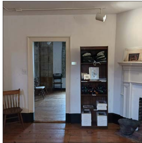
78-4: Cracked paint and plaster around door frame
