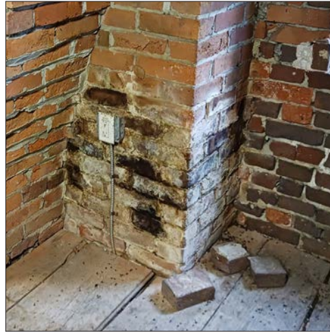
101-2: Efflorescence and damaged bricks in the chimney as seen at the attic level.
