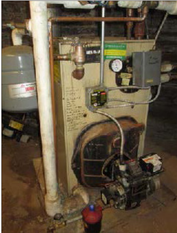
110-1: Oil fired boiler
