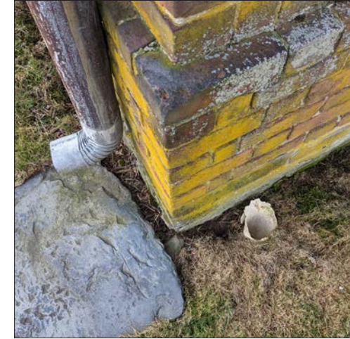
39-5: Vegetation growing on water table and side of wall. PVC pipe should be removed if it is not performing a useful service.
