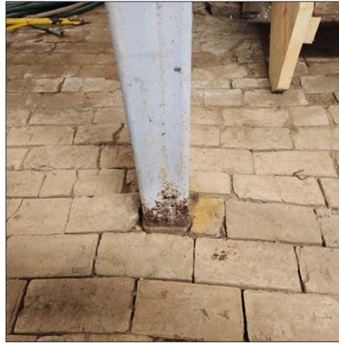
59-2: Steel columns at basement level.
