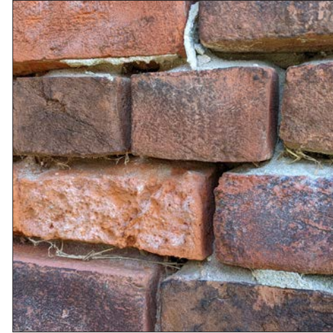
54-5: Mortar and brick detail. Some bricks are spalling and mortar is deteriorating.
