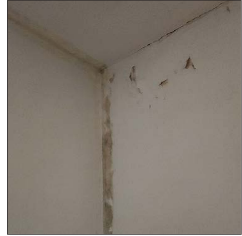
78-5: Peeling paint at corners of wall and ceiling; strip along wall edge removed to show previous paint finishes.
