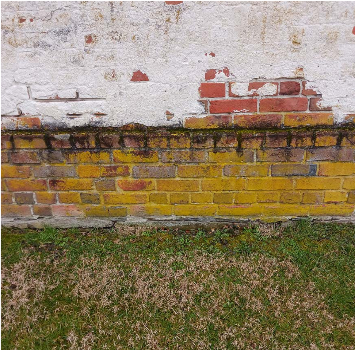
50-1: Stucco coating on brick is deteriorating; some bricks are spalling.
