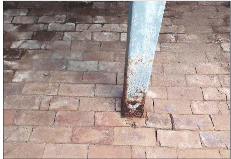
104-4: The only structural defect identified was the rusting at the base of the new steel columns in the basement.
