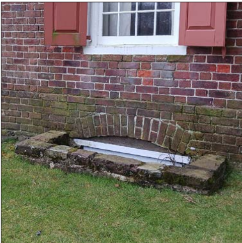
39-3: Plants should be removed from window wells and any leaks should be repaired to avoid water infiltration into the basement.
