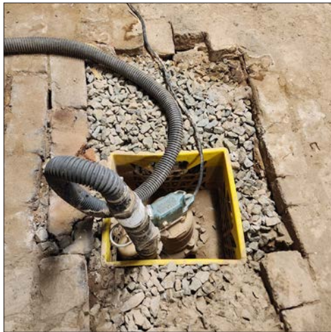
59-4: Existing sump pump.
