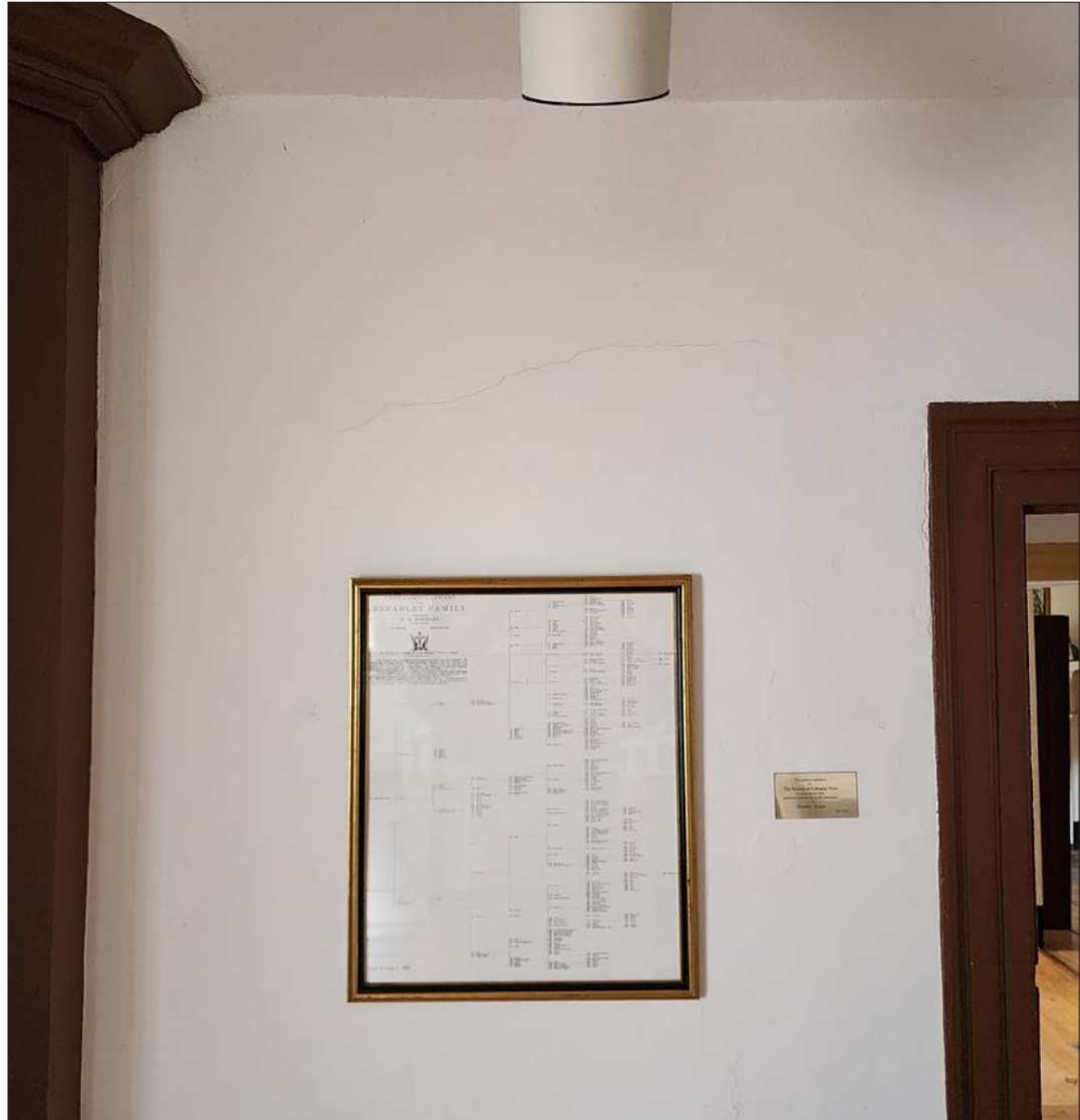
64-3: Plaster at walls is cracking and needs to be repaired.
