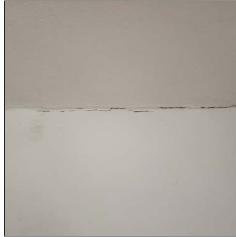
98-2: Cracked plaster at meeting of ceiling and wall
