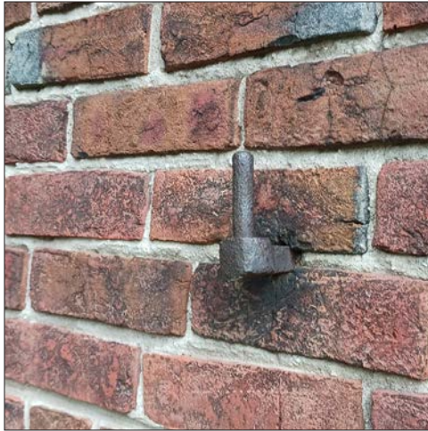
54-1: Miscellaneous metal object embedded in wall; location not associated with window opening or doorway. Function unknown, corrosion could cause damage to mortar and brick face.
