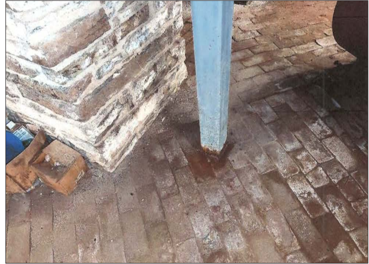
104-2: The only structural defect identified was the rusting at the base of the new steel columns in the basement.
