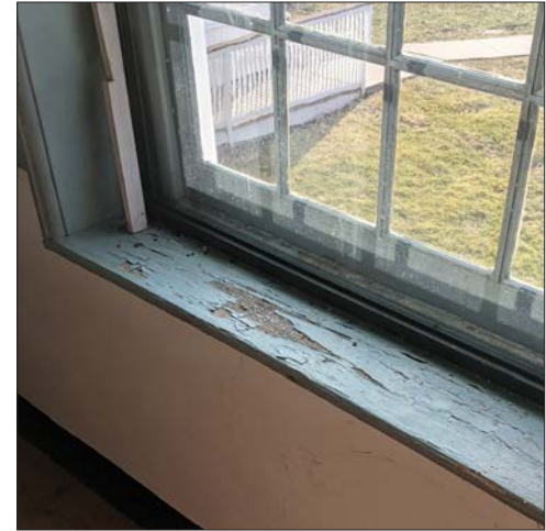
94-3: Paint peeling at window sill.
