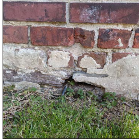
54-4: Gap at base of exterior masonry wall. Stucco coating has been damaged.
