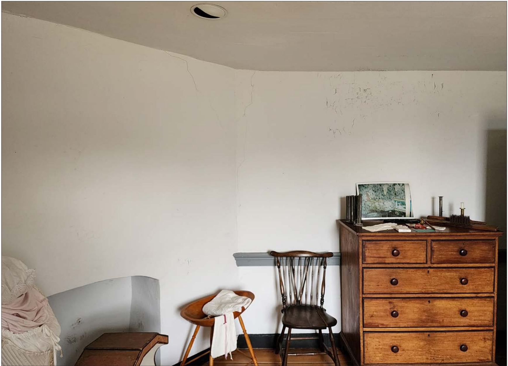
95-1: Plaster cracking above wall. Image placed on period furniture shows room prior to 1999 work.
